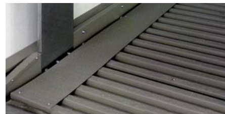
Catwalk on trapez. sheet for more walking comfort
